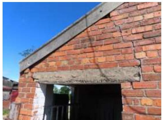
Large crack stemming from lintel to verge
