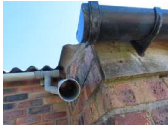
Downpipe missing from front left corner
