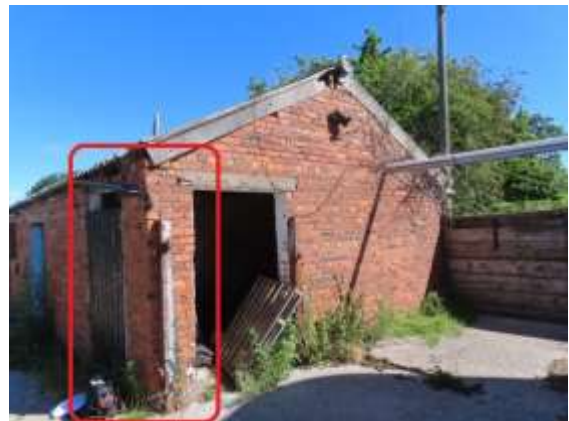
Damage and rotational movement to front right corner
