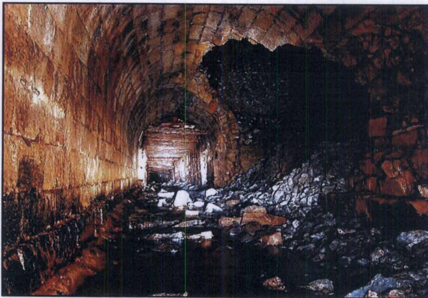
Well-constructed roadway with collapse
