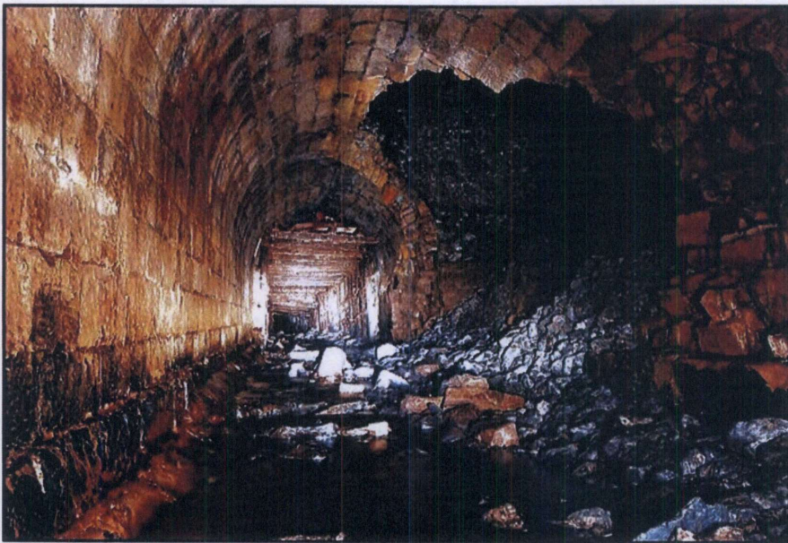
Well-constructed roadway with collapse
