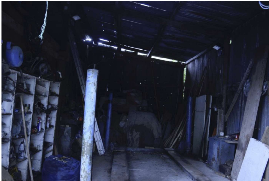
Figure 4.8. Showing gaps at the eaves.
