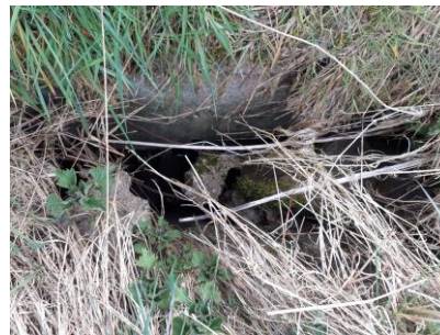
Figure 29: Collapsed culvert in field at TN25
