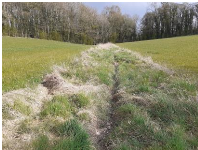
Figure 28: TN24 brook running under field in a partially collapsed culvert of TN25
