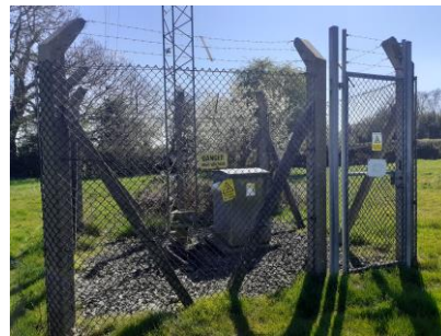
Figure 37: Fenced off electrical conductor structure associated with the sub-station and mast
