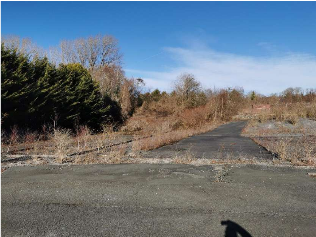
Plate 9. – Hardstanding surfacing and overgrown vegetation
