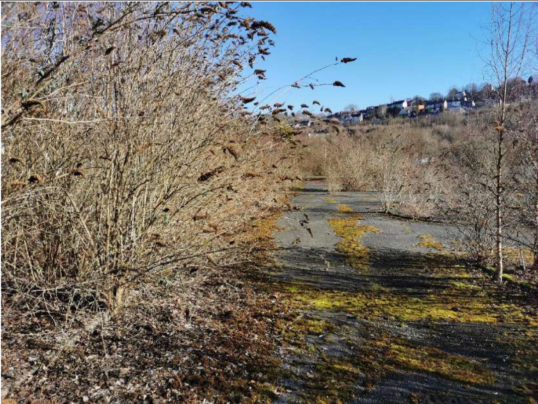
Plate 4. – Hardstanding surfacing and overgrown vegetation
