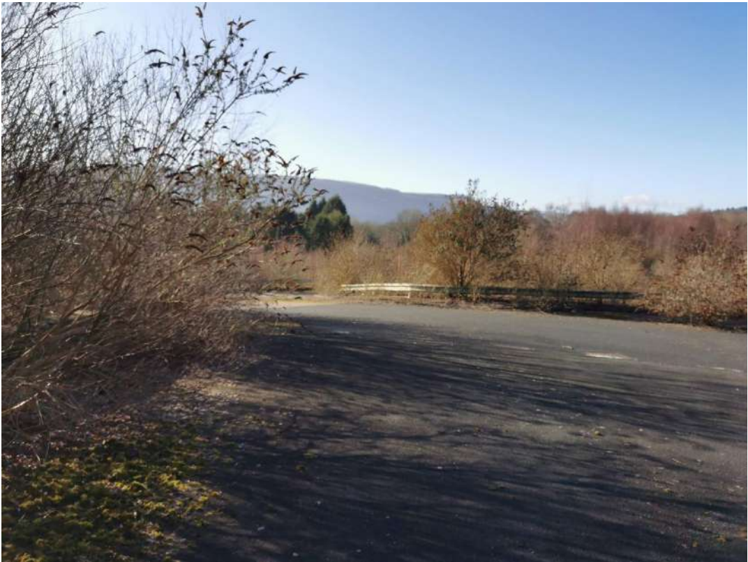
Plate 15. – Hardstanding surfacing and overgrown vegetation
