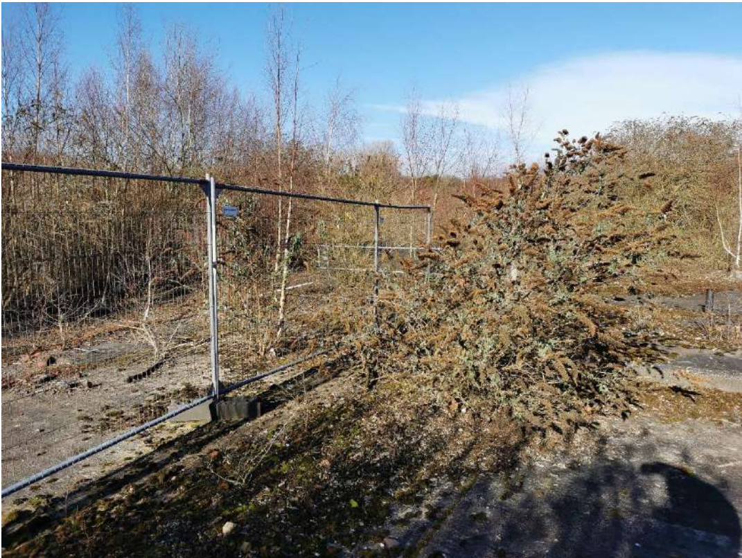
Plate 25. – Hardstanding surfacing and overgrown vegetation. Localised fencing.
