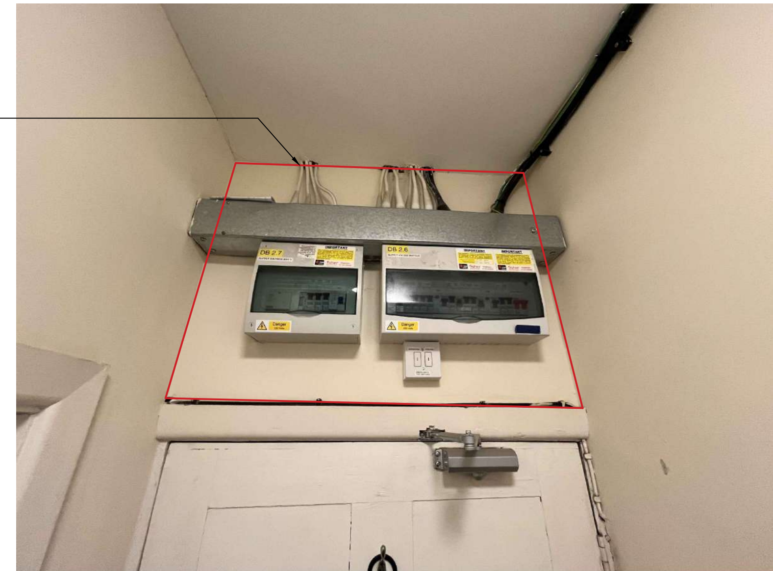
Image 01 Electrical box viewed from inside KG13 to be boxed up as it is above emergency escape route
