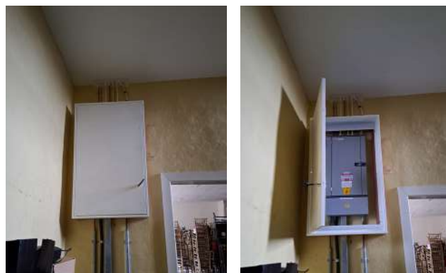
Examples of proprietary distribution board enclosures.
