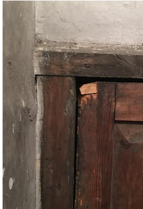
Poor condition of door T4
