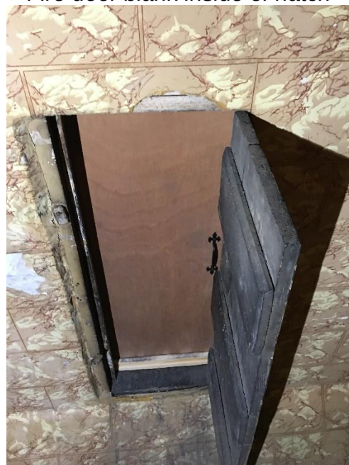
Fire door blank inside of hatch
