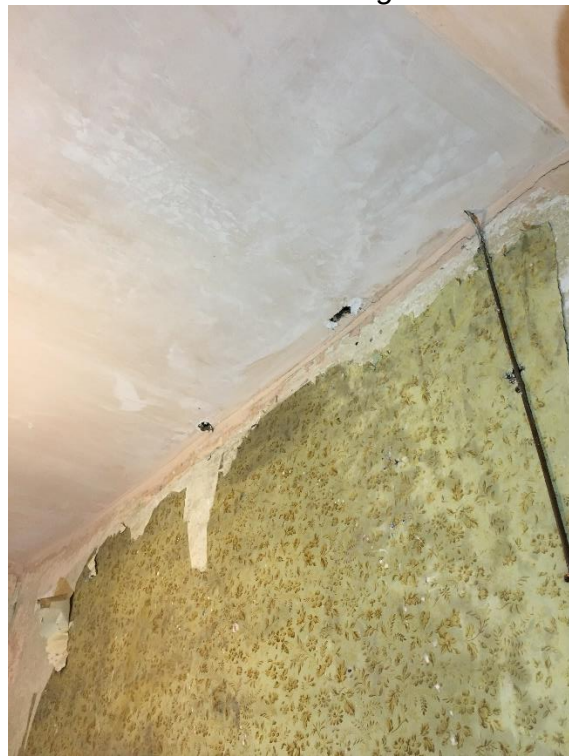
Holes in ceiling
