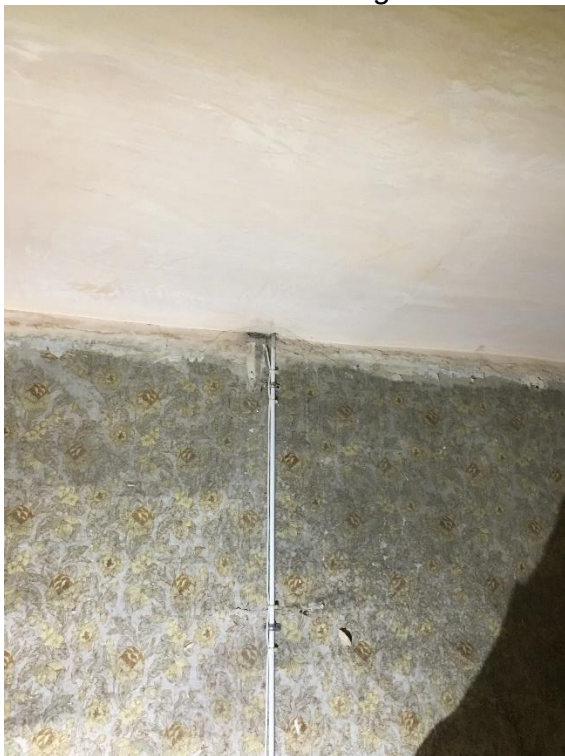
Holes in ceiling
