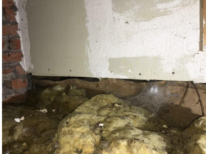
Underside of Barrier not sealed
