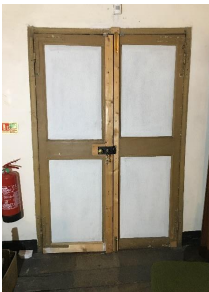
Door T18 with intumescent covering and narrow stiles and rails
