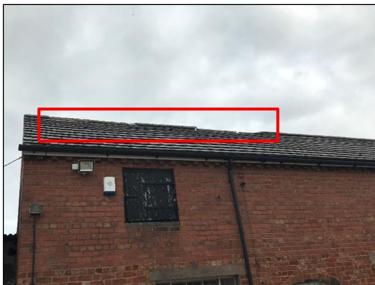
Plate 12. Missing and lifted ridge tiles at western end of Barn
