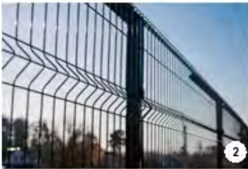
BOUNDARY SECURITY FENCE 2.4m High Paladin Fence
