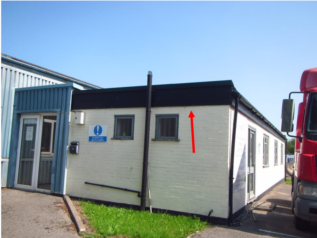
Photograph 16 – Southern aspect of Building 4, arrow pointing to gap in barge board.
