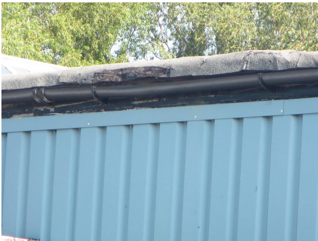
Photograph 13 – Slightly lifted roofing felt on Building 3.
