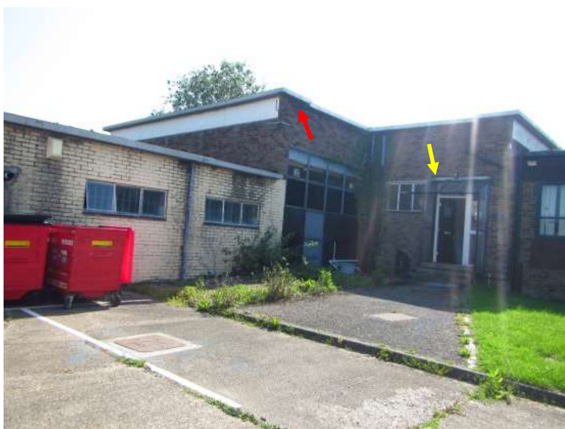
Photograph 4 – Red arrow shows location of gap in brickwork. Yellow arrow shows the location of Roost 1; beneath the lead flashing of the porch.
