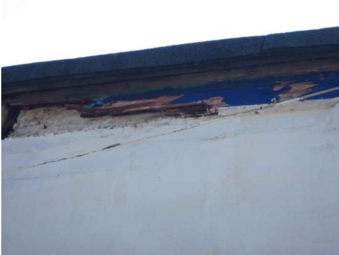
Photograph 9 – Broken fascia board on Building 2, western aspect.
