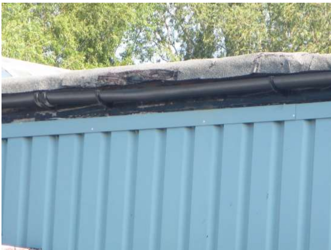
Photograph 13 – Slightly lifted roofing felt on Building 3.
