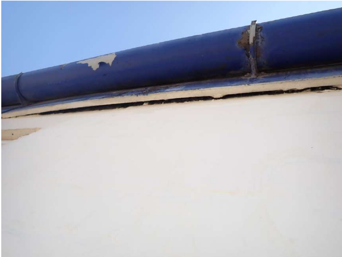
Photograph 11 – Gap under fascia board on Southeastern aspect of Building 3.
