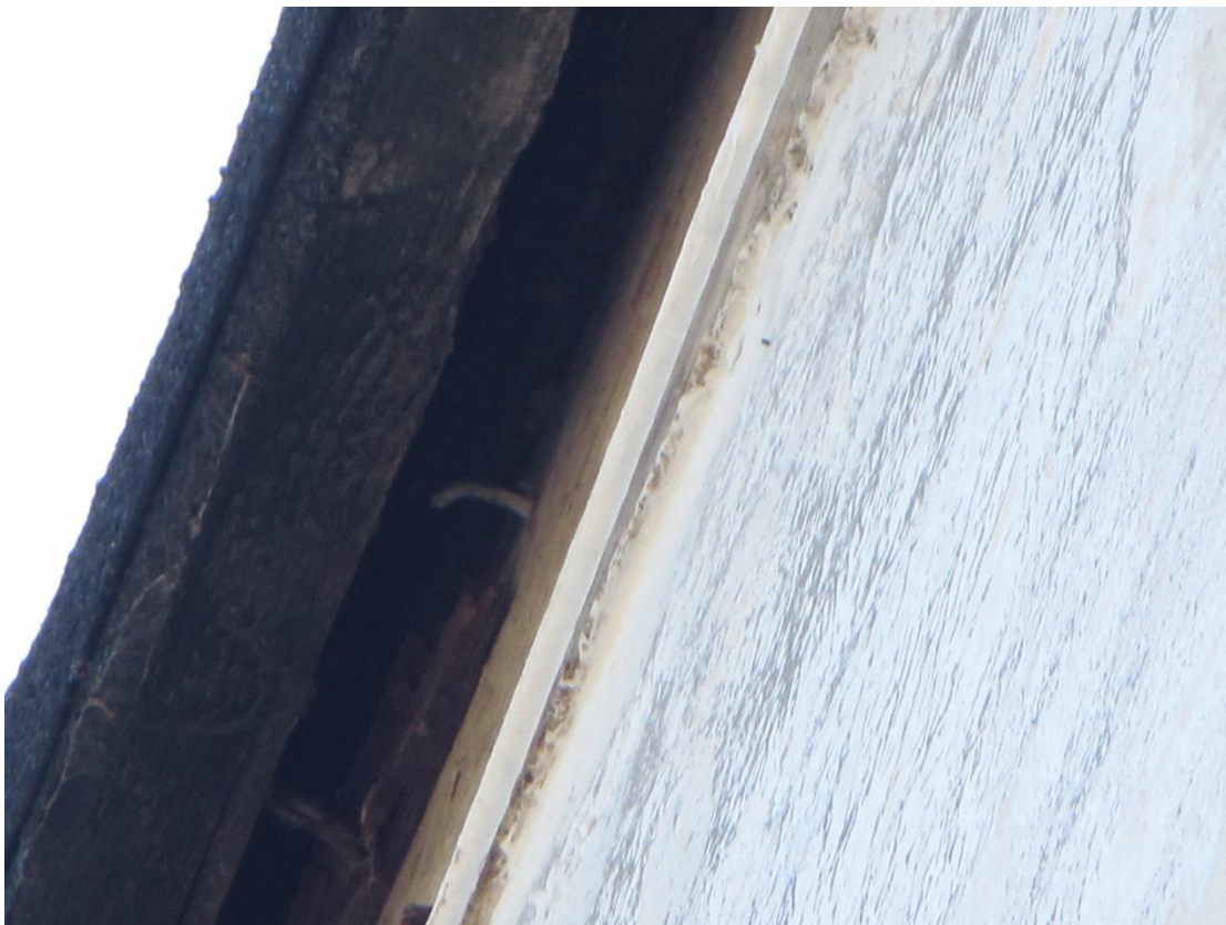
Photograph 8 – Gap between overhanging roofing felt and fascia board on western aspect of Building 2.
