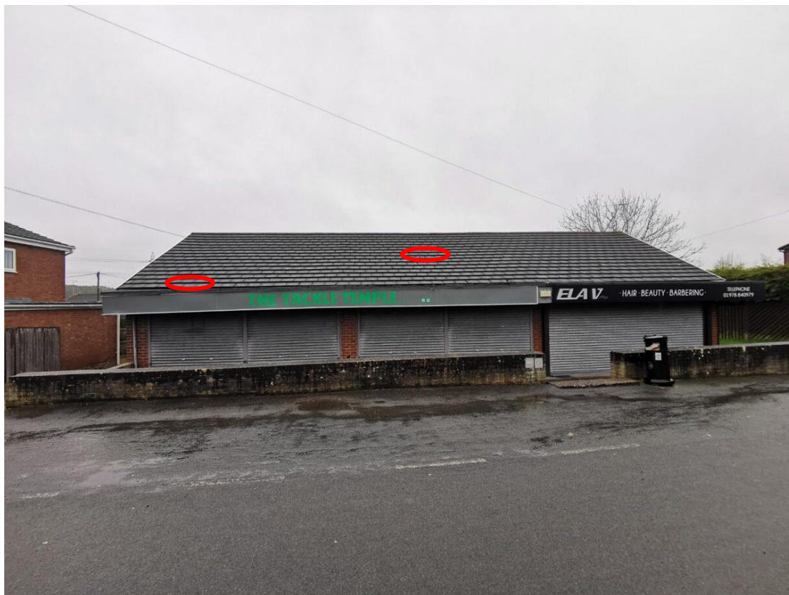
Plate 13 - A view showing the locations of PRF's in the form of slightly lifted roof tiles (red circles).
