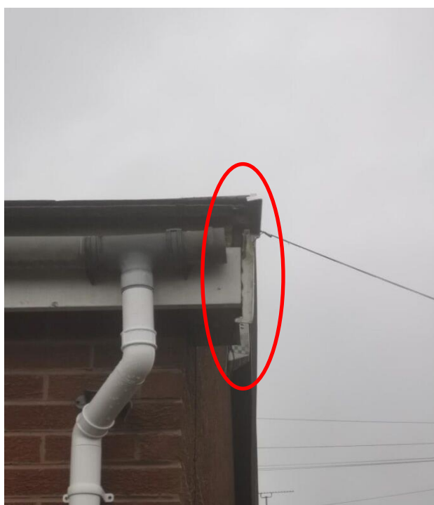
Plate 10 – A PRF consisting of a gap behind the fascia board on the north-eastern extent of the building.
