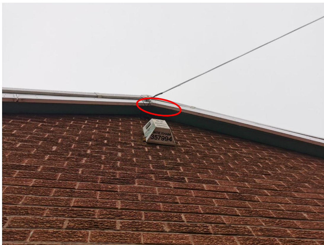
Plate 12 - A PRF consisting of a lifted fascia board.
