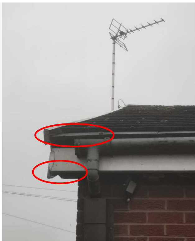
Plate 11 - PRFs under the verge roof tile and behind the fascia board on the south-eastern extent of the building.
