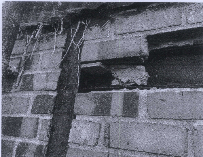
A1.7 Plate 7: Dislodged brickwork showing voids and crevices
