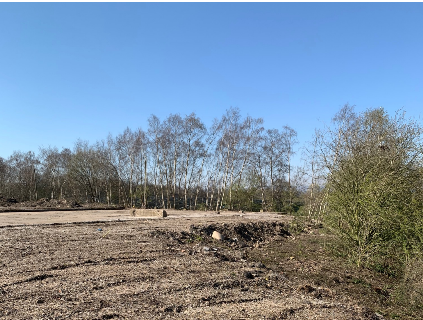
Purifier bases - Exterior Image
