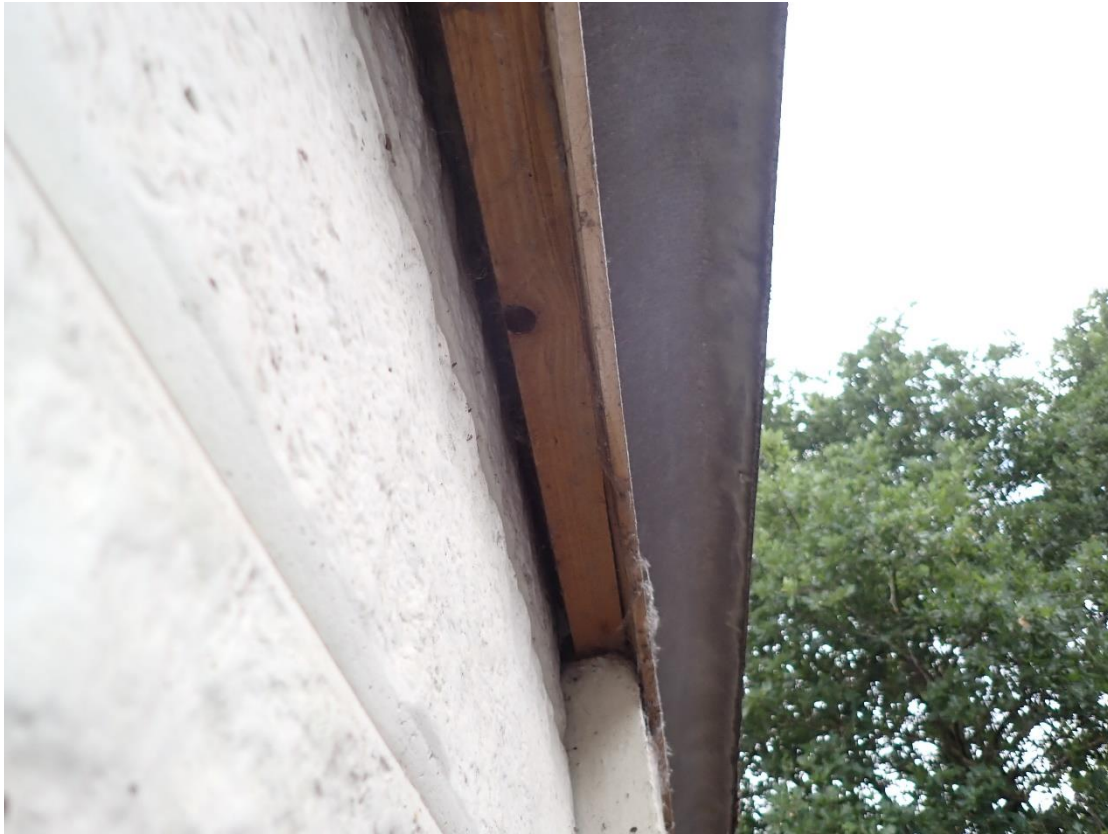
Photograph 3 – gap beneath timber barge board on northeast aspect.
