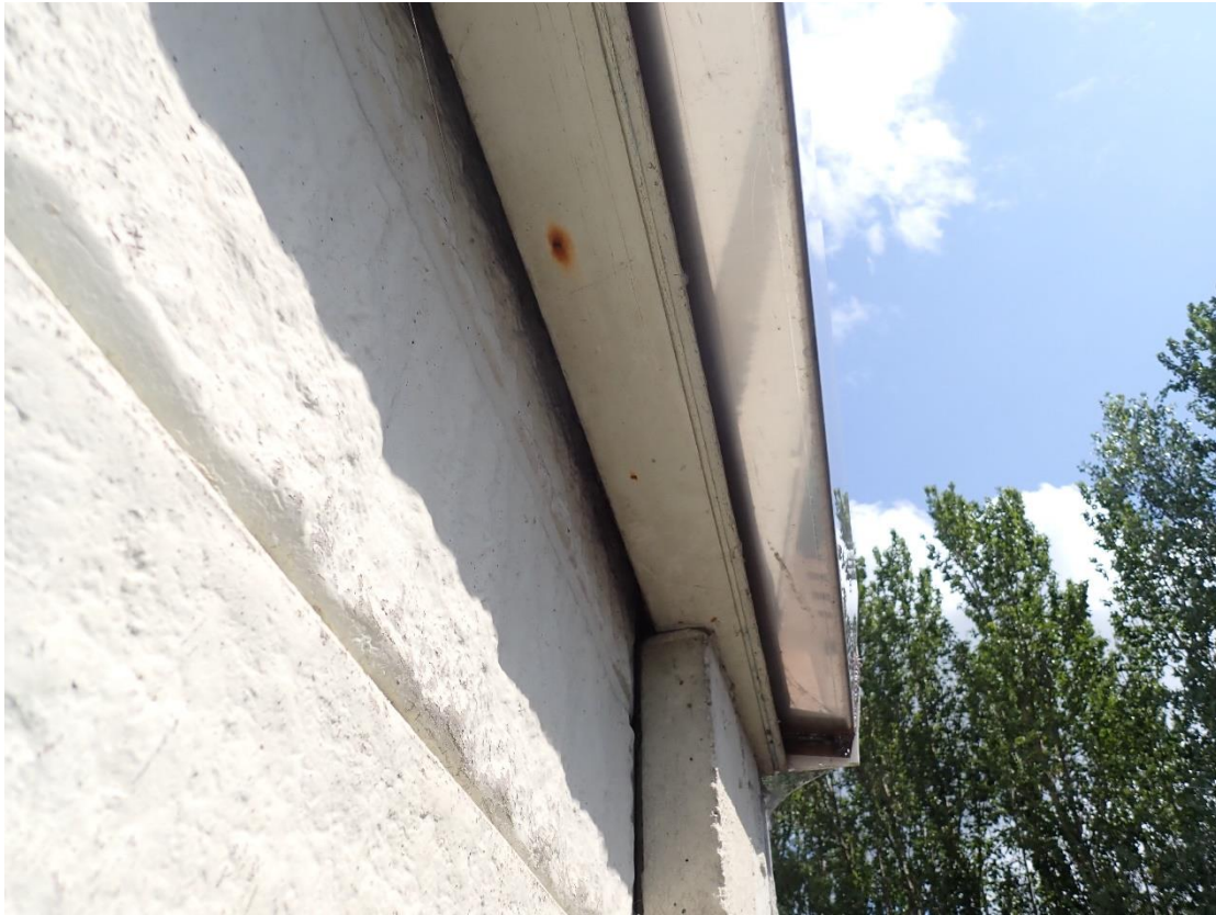
Photograph 9 –gap between timber soffit and concrete façade on south aspect of building on site.
