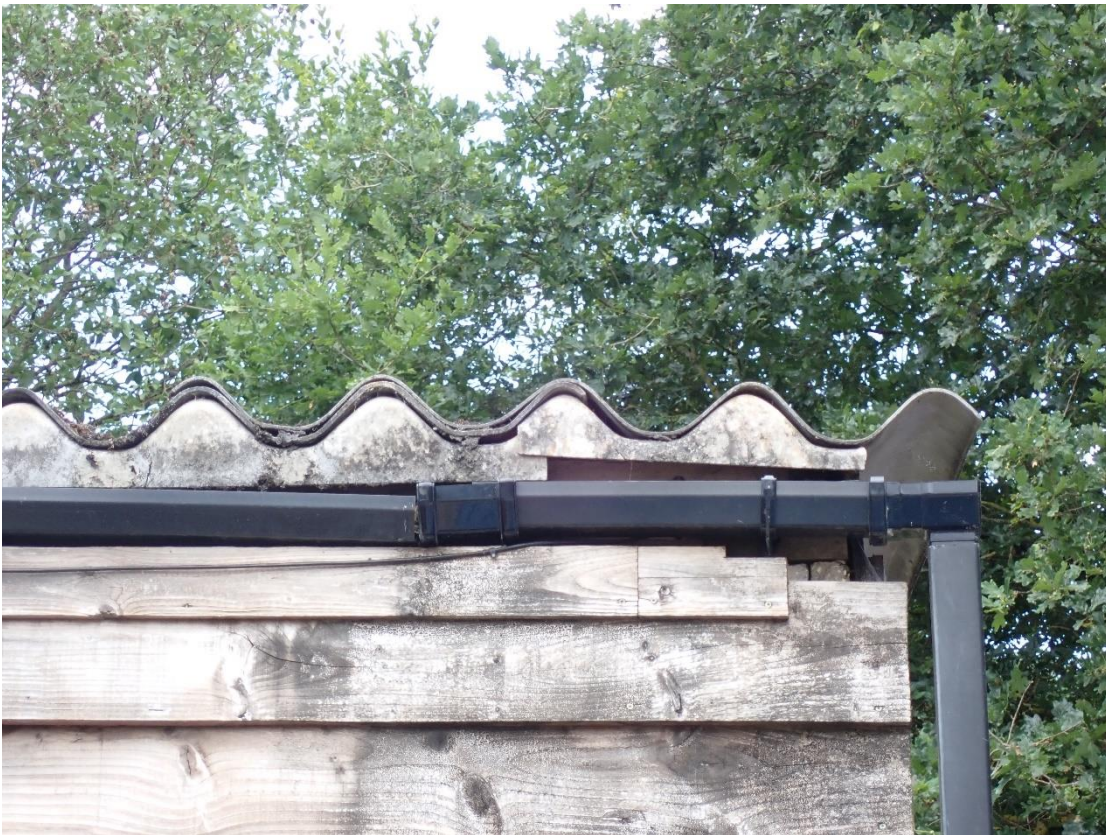
Photograph 2 – southeast aspect of building 1 showing lifted corrugated asbestos sheeting.
