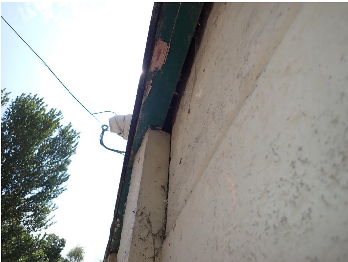
Photograph 8 – gap beneath timber barge boards on northeast aspect of the building on site.
