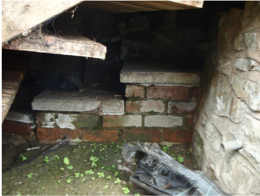
Defunct brick/ patio slab steps located underneath the raised wooded decking at Target Note 2 .
