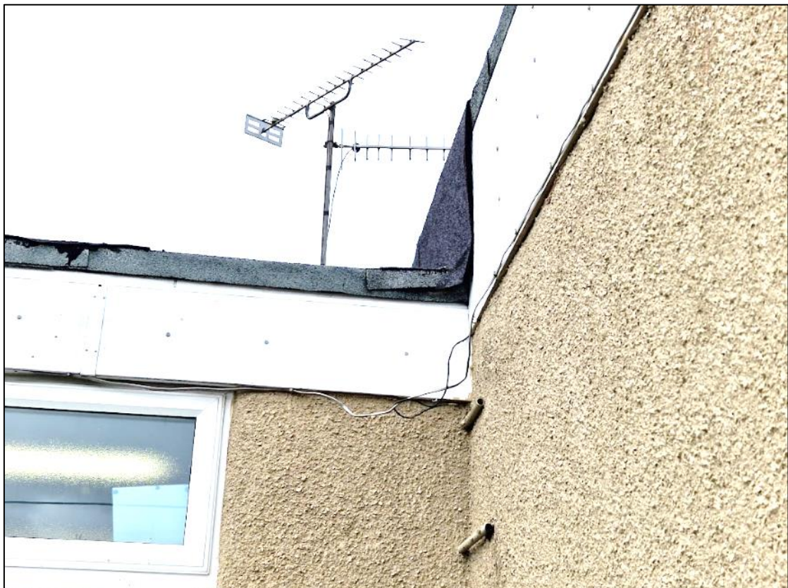
Plate 2 – Minor lifting of the roofing felt on B1
