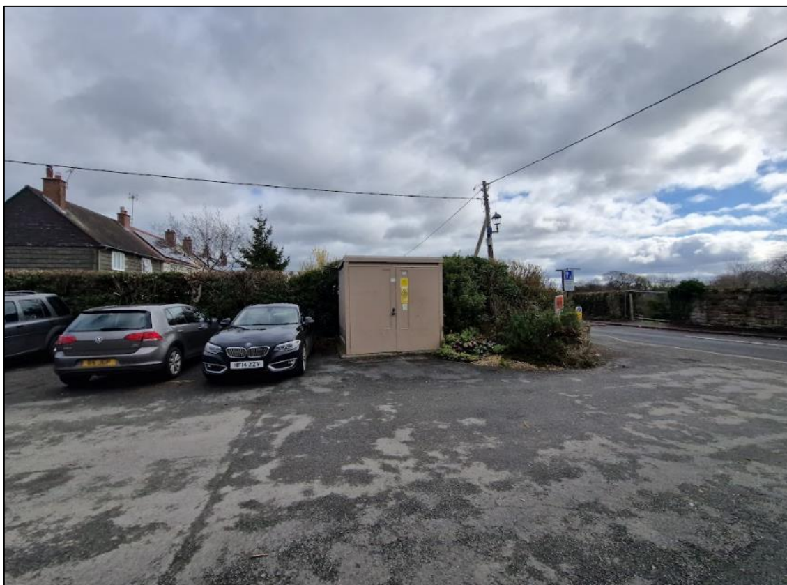
Plate 7 – Building 5 – Electrical unit
