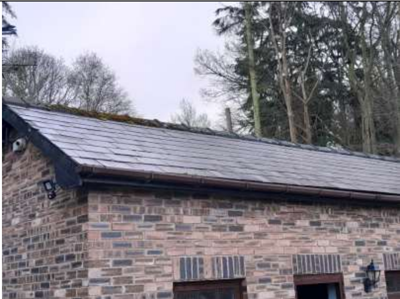
Figure 8 - damaged tile towards the northern gable is shown to still be present and does not create a roosting feature.
