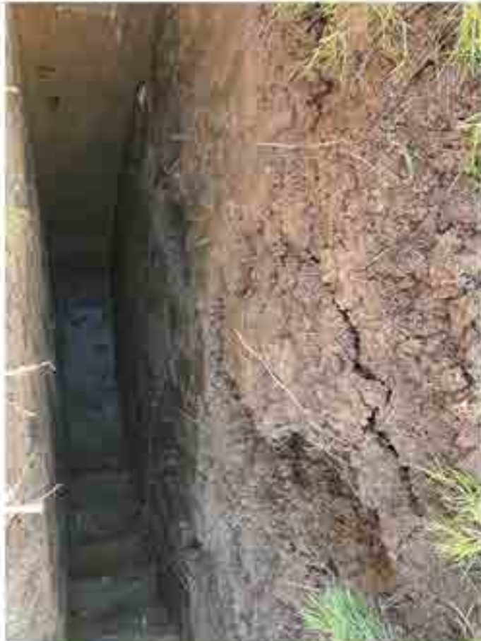
TP104 Face A close up
