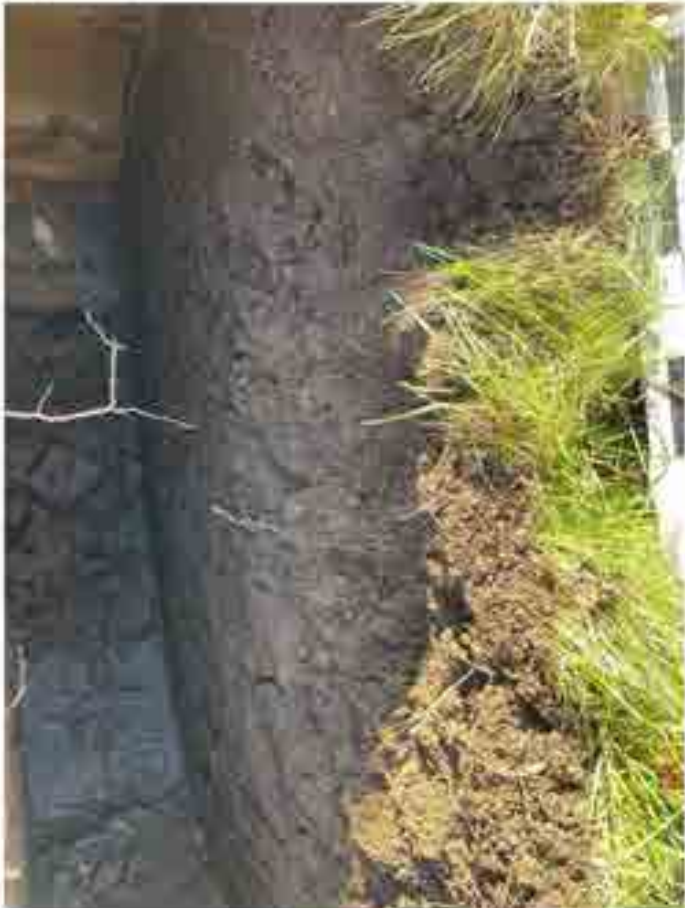
TP101 Face A close up
