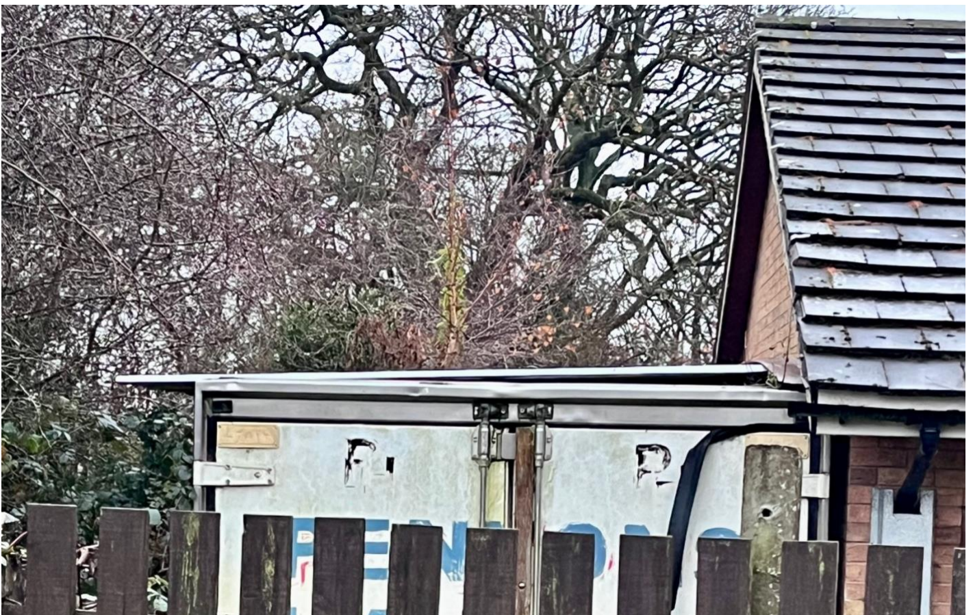
Photo 4 – Note the temporary attempt on the roof of the container trying to keep the rain out
