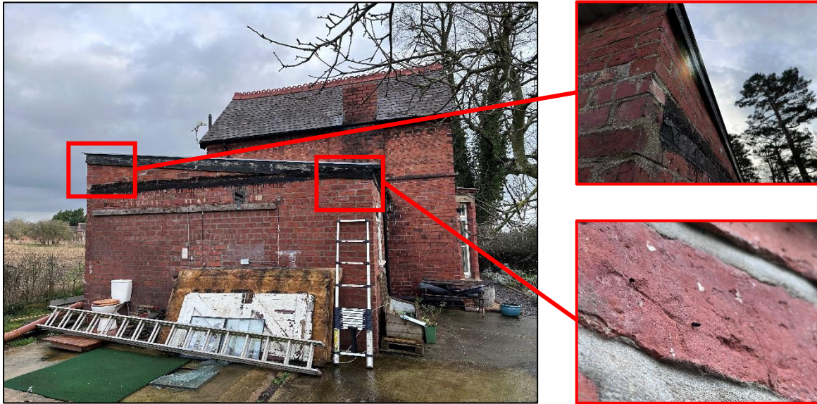
Figure 8: Showing the location of droppings identified under the fascia board.
