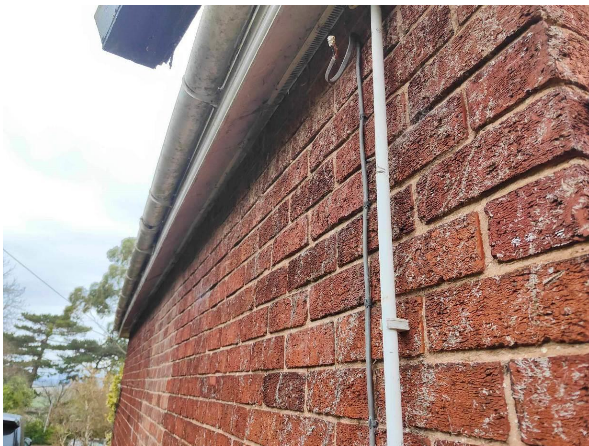
Pointing and soffit.
