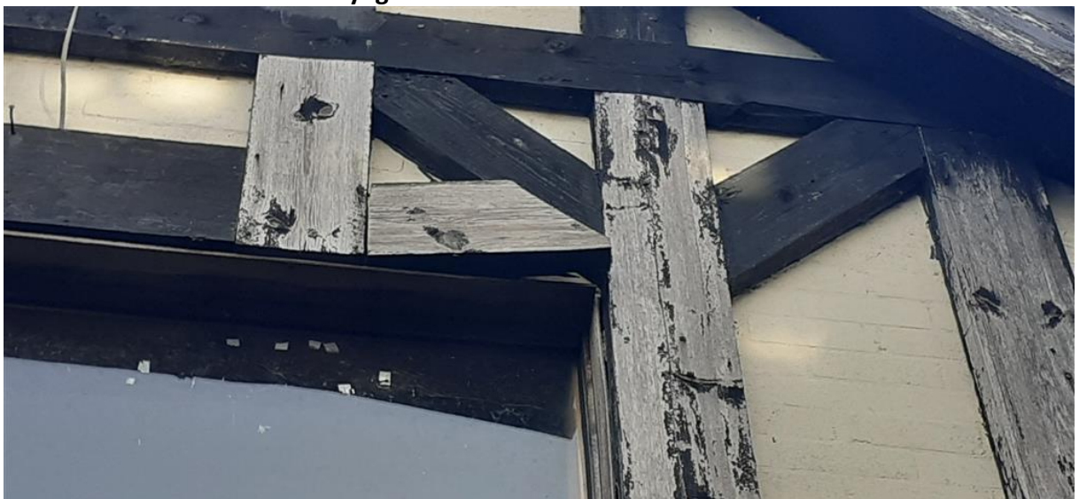
Plate 6: View of the loose piece of the façade timber framing -eastern elevation.
