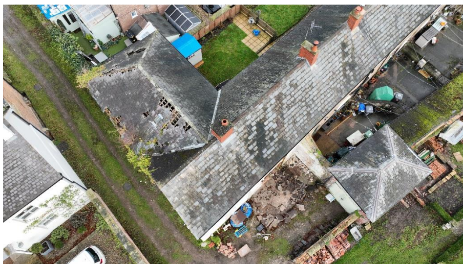
Figure 6. Damage to roof seen in December 2023
