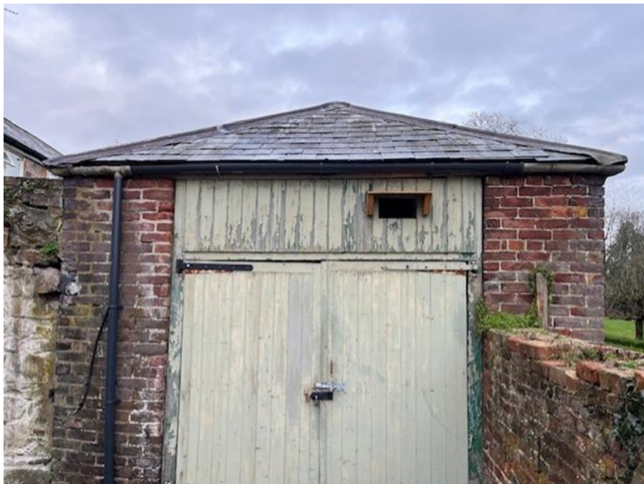
Figure 11. Letterbox opening for LHS bats in garage
