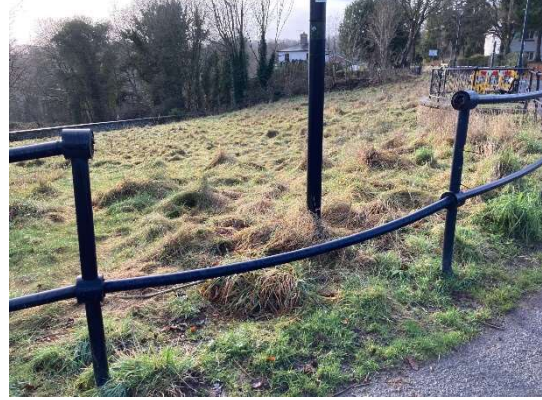
Figure 2: Example of failed elements
