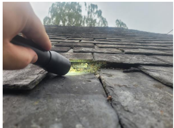
P6: Example of a missing slate with cobwebs inside
