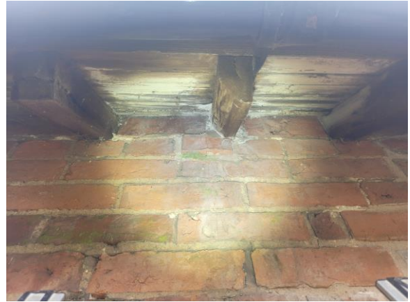
P8: Example of the obstructed eaves and sarking
