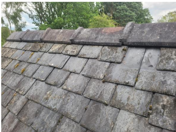
P5: Example of the ridge and roof-tiles, with slipped slate
