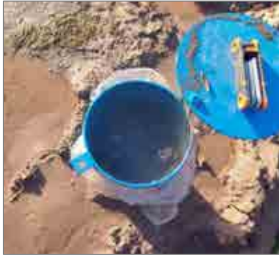
Photograph 1 – Flooded upstanding cover on BH102
