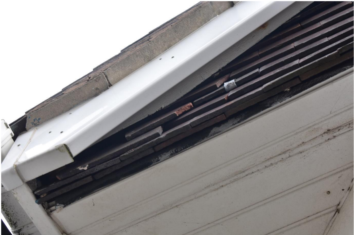
Figure 3.6: The gaps present on the hanging ceramic tiles fitted onto the dormer window.
