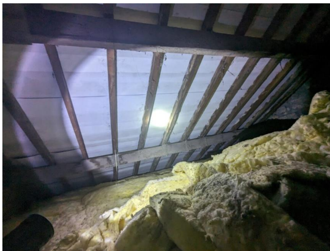
Plate 6 – The loft space of B1 with the piled insulation in one corner.
