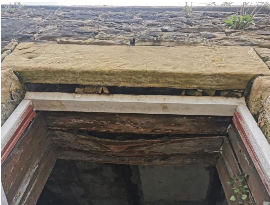
Plate 13 – Void behind window lintel of B2.
