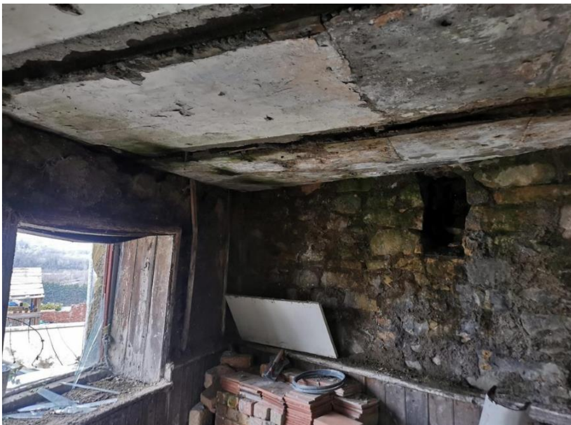
Plate 11 – Internal view of B2 with voids in the wall and ceiling visible.
