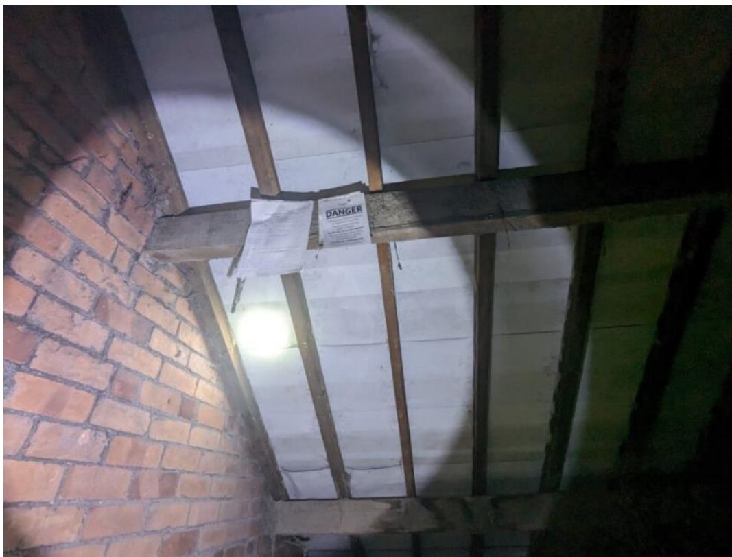
Plate 7 – ‘Danger’ sign attached to a purlin within the loft space of B1.
