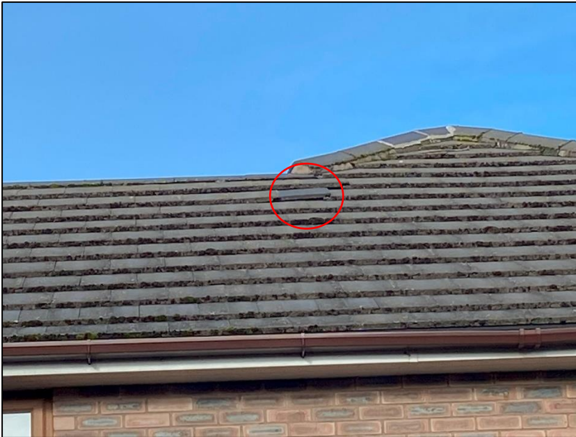
Photograph 9 showing the slipped tile
