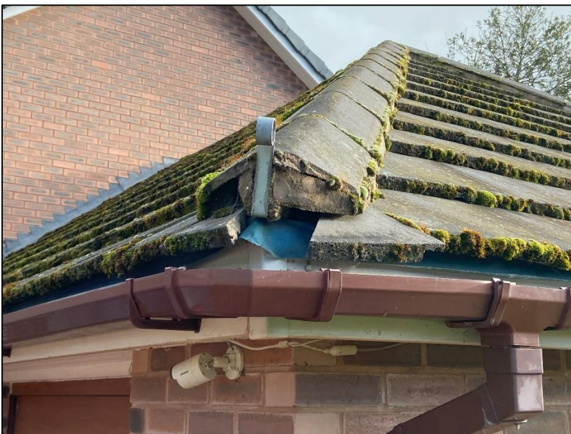
Photograph 10 showing the cavity in the garage roof
