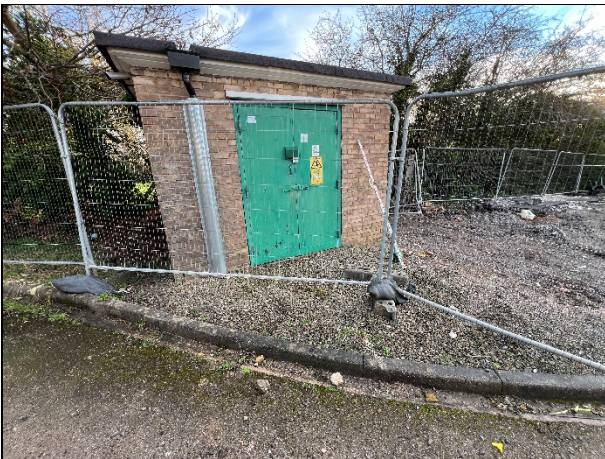
Photograph 1: South west side and access point to electricity sub-station. Photograph taken by Coopers on 2 nd February 2024
