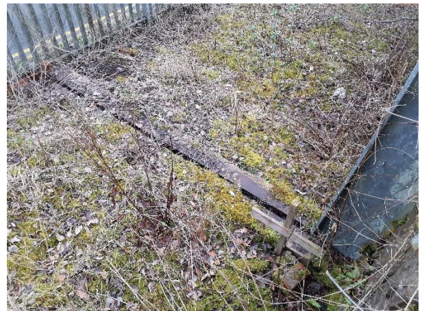
FIGURE 4.5: AMPHIBIAN EXCLUSION GRILLE AT THE NORTHERN END OF THE FENCING, ADJACENT TO BLAST ROAD
