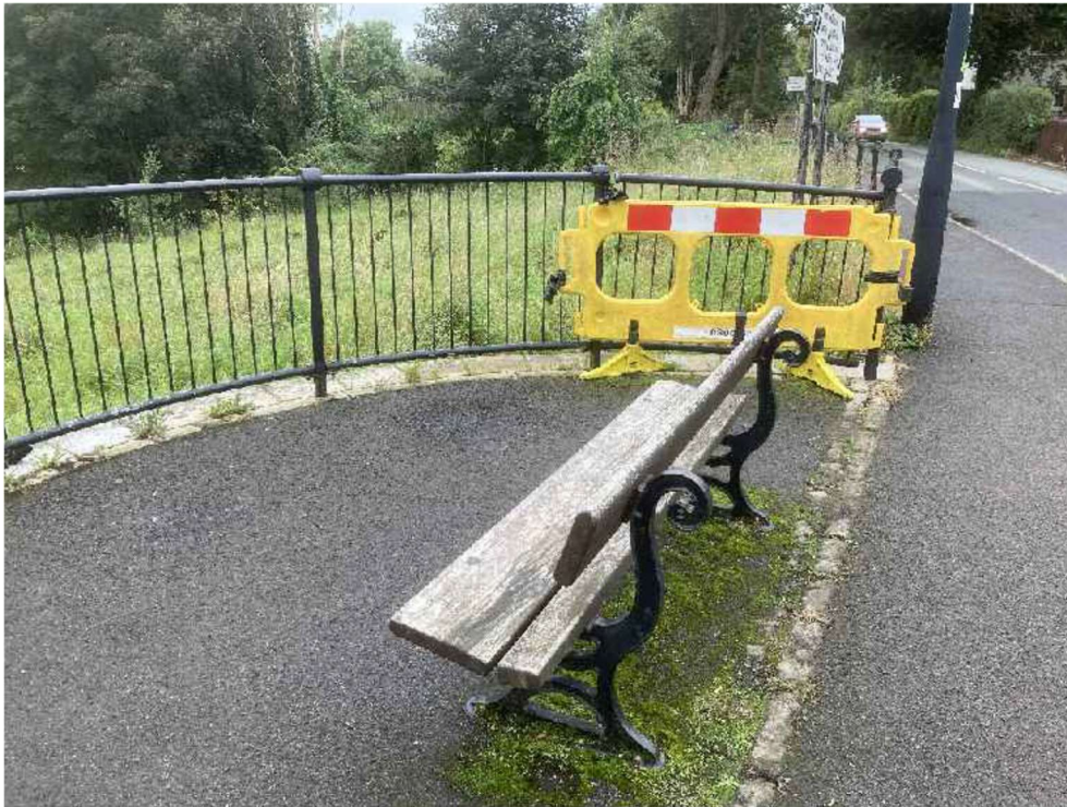
Figure 4 - Photo showing the existing railing arrangement at the viewing area. A temporary barrier is in place where a section of this fencing has failed.
