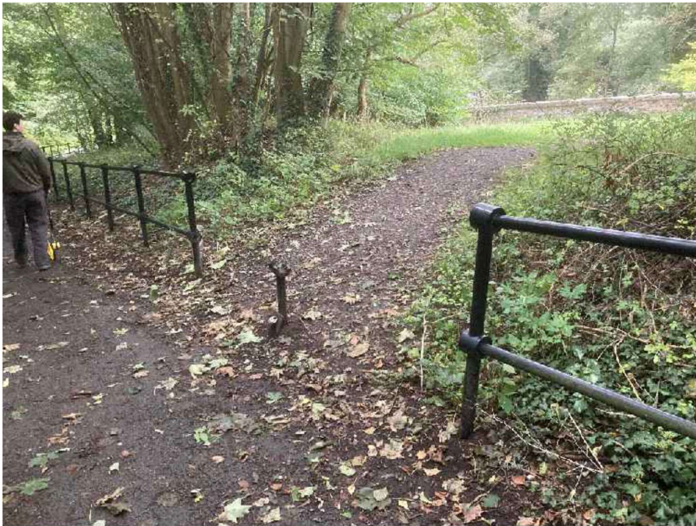
Figure 5 - Photo showing a section of the existing railings which has failed and enabled unauthorised access to land above the tunnel portal.
