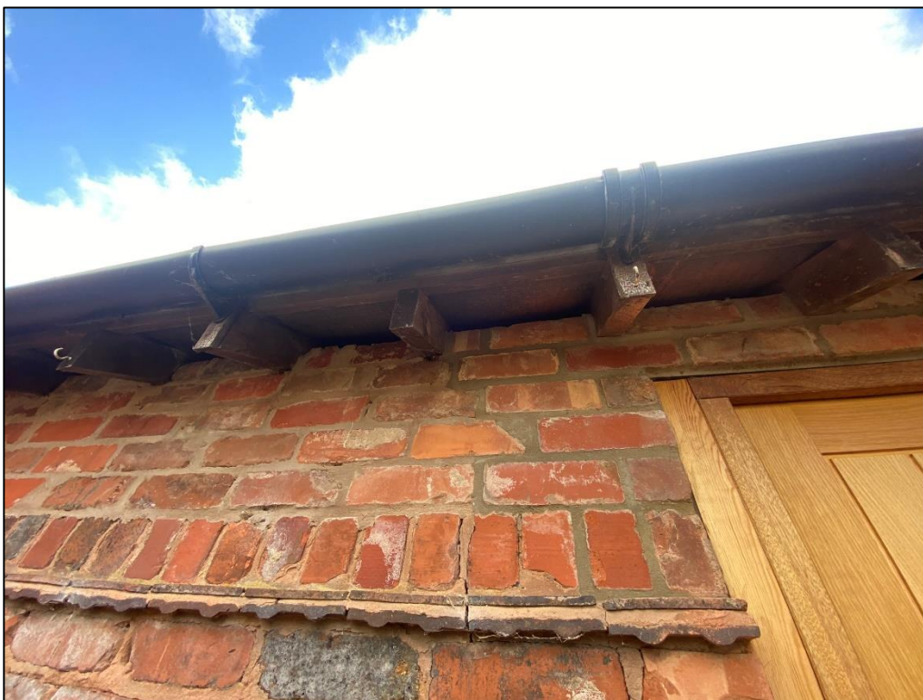
Plate 13 – Open eaves at the adjoining section of the building
