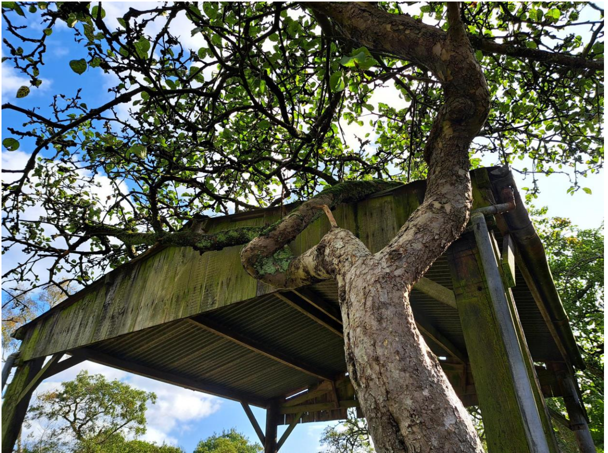
Figure 4 T30 leaning on the dutch barn proposed for removal, effectively propping up T30
