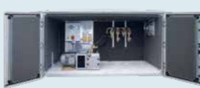
Concrete external cabinet
