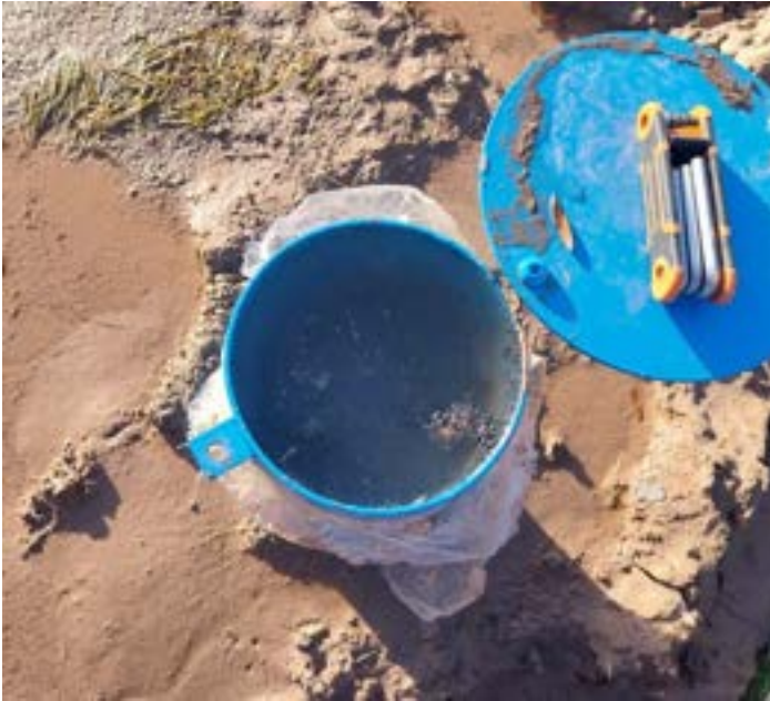
Photograph 1 - Flooded upstanding cover on BH102
