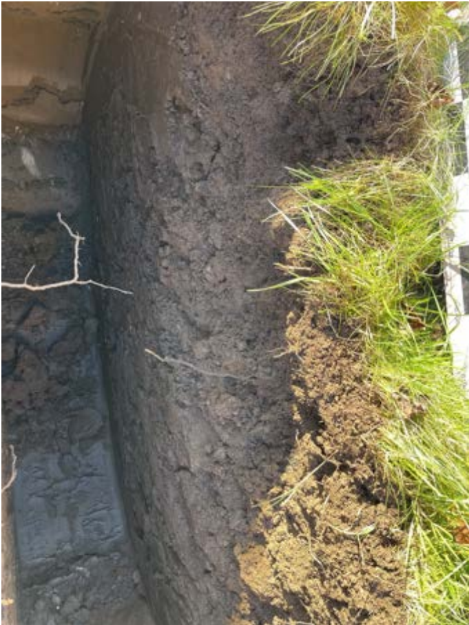
TP101 Face A close up
