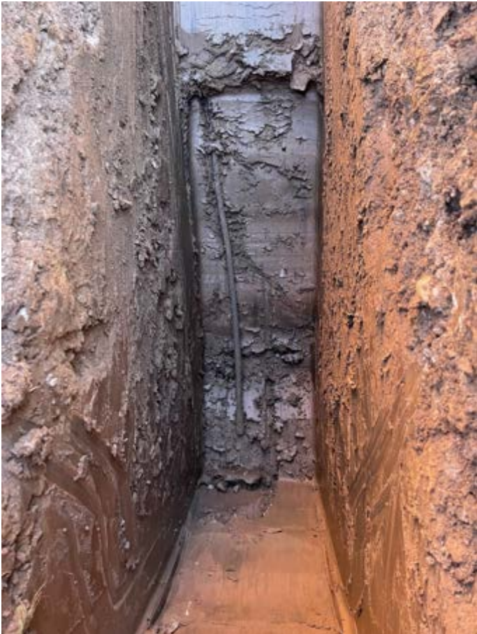
TP105 wire at base
