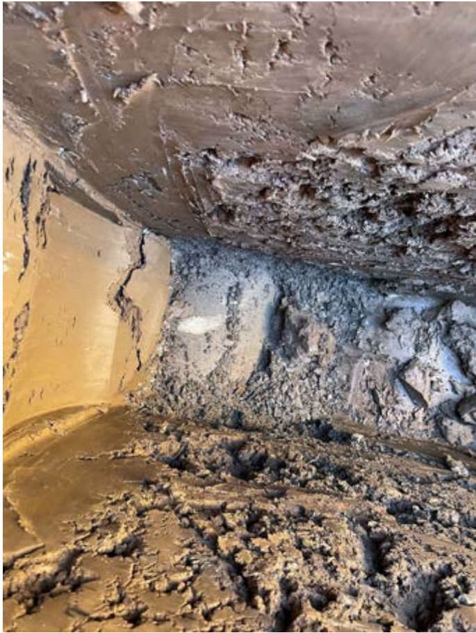
Concrete utility at base 1
