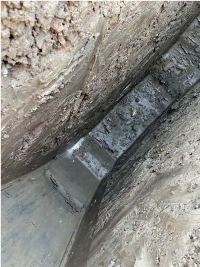
Concrete utility at base
