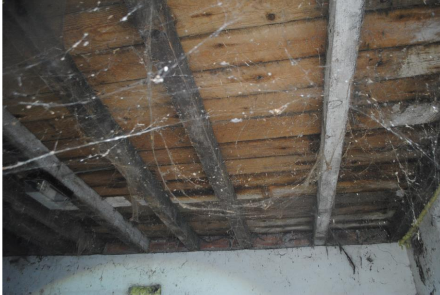
Figure 4.7; Cobwebs under mezzanine floor
