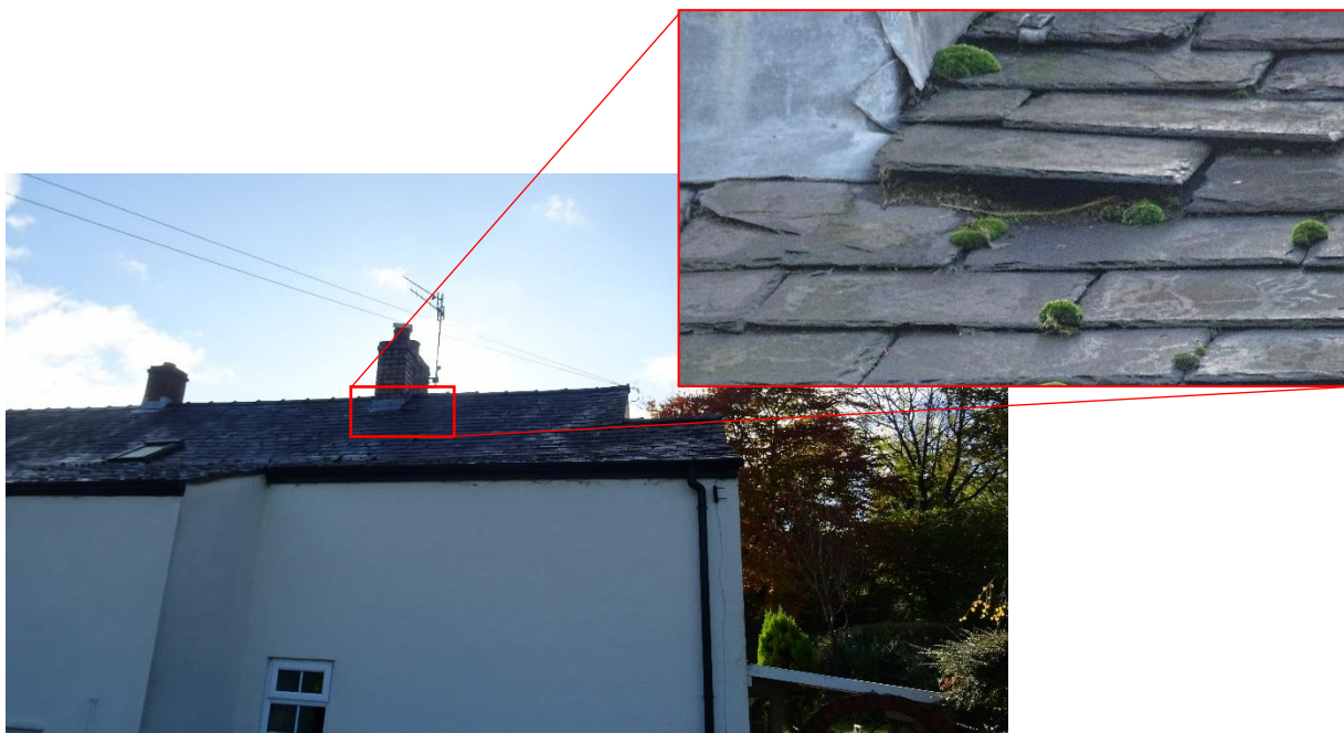
Figure 4.5. Small gap beneath raised tile
