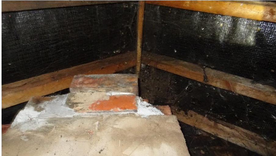
Figure 4.6. Heavy cobwebbing around ridge in western loft
