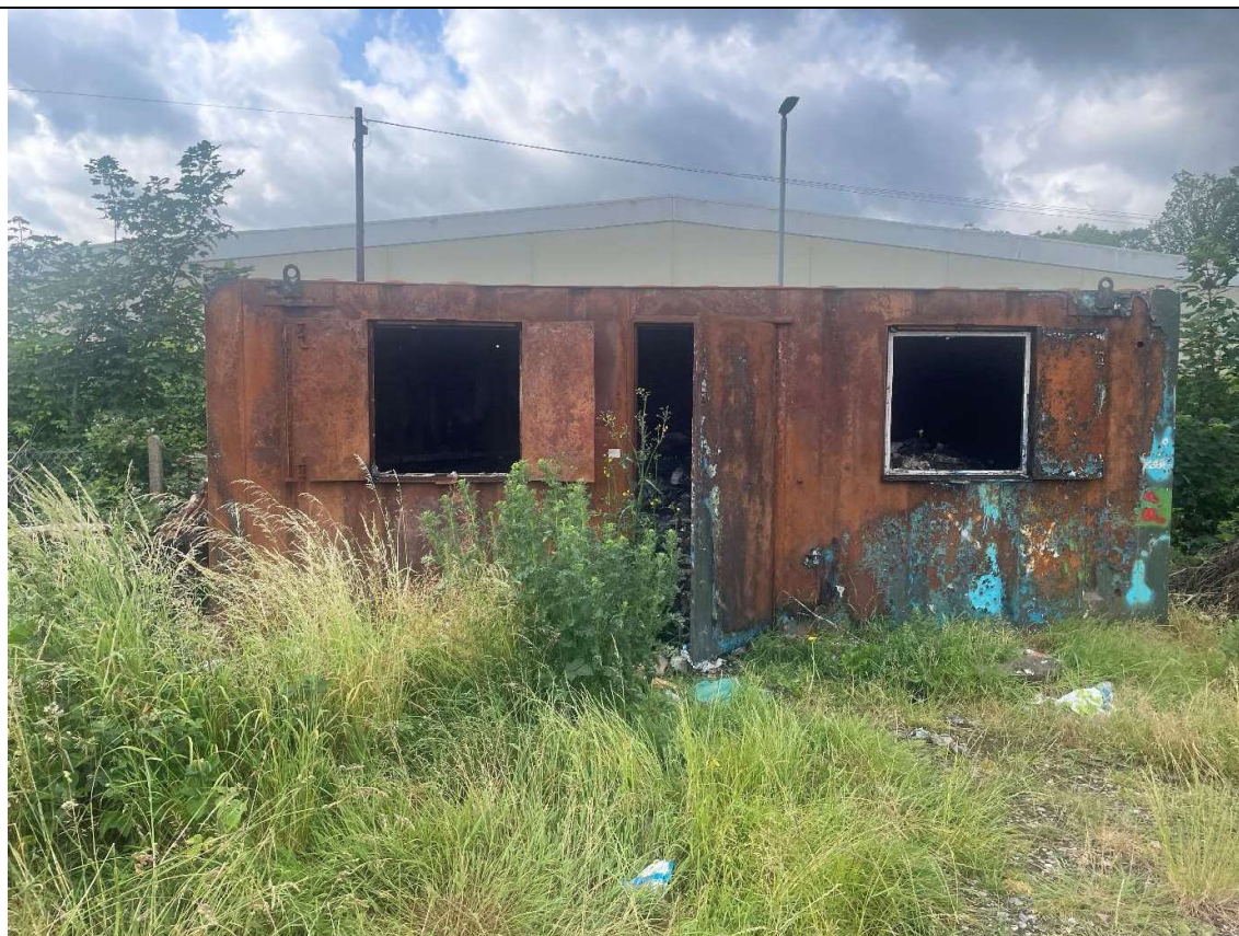
Photo 5 – Old container with evidence of fly tipping inside located at the south of the site.
