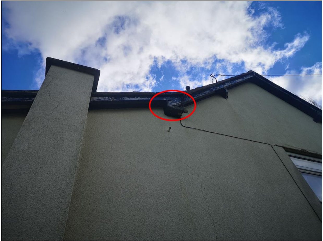
Figure C7.3: Emergence point from soffit on western elevation of the dwelling
