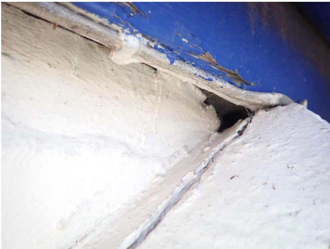
Photograph 16 – Hole under fascia over brick pillar on Southwestern aspect of Building 4.
