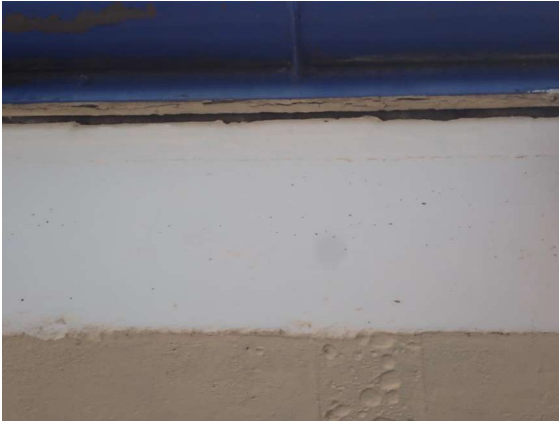
Photograph 15 – gap under fascia board on Southwestern aspect of Building 4, above the roller shutters.
