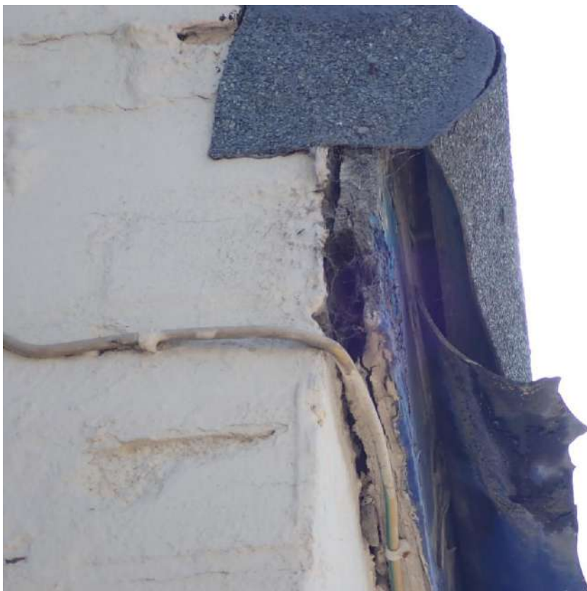
Photograph 12 – Gap towards end of guttering on Southwestern aspect of Building 3 with raised bitumen felt.
