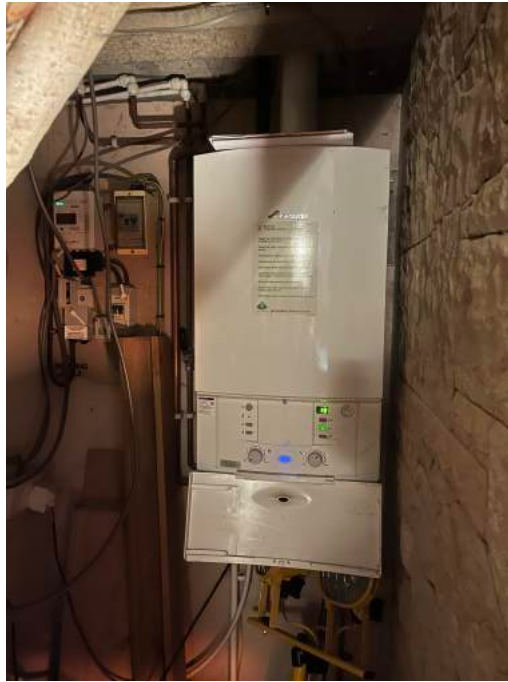
FIGURE 2: Image of the existing boiler.
