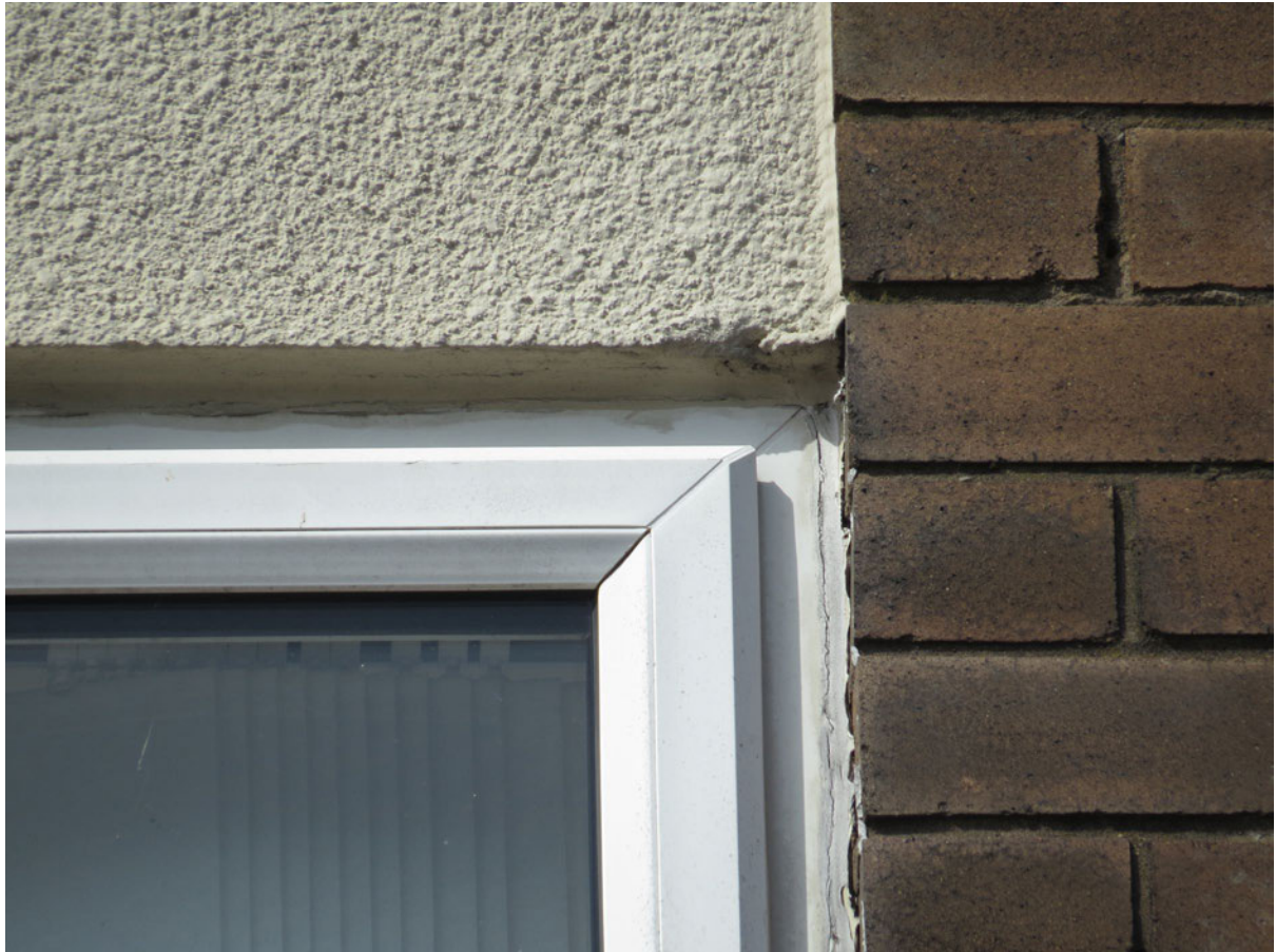
7 – Window and door frames are sealed tightly into brickwork with no suitable gaps.
