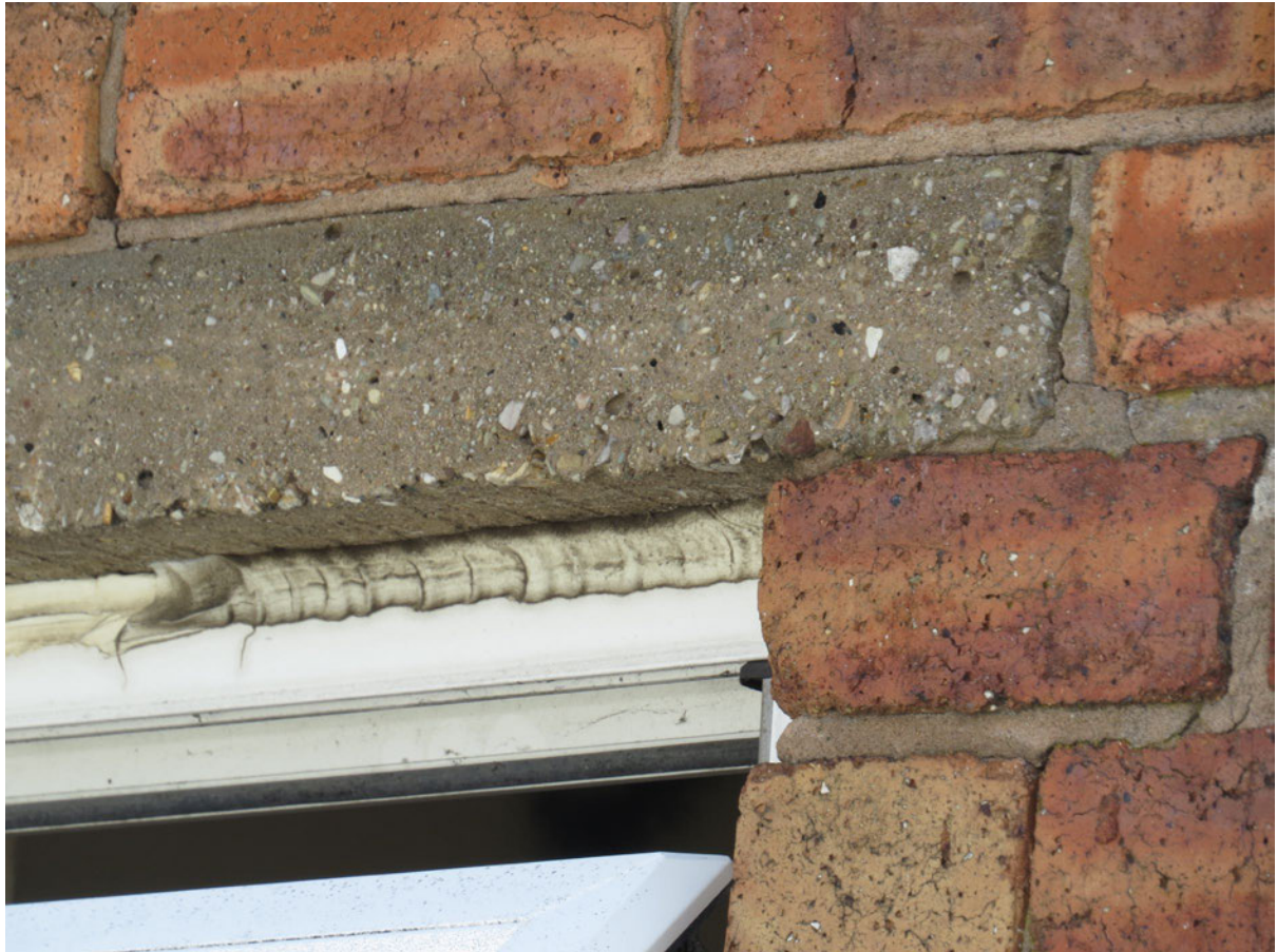
5 – Lintels are concrete, and are fixed into the walls with no suitable gaps.
