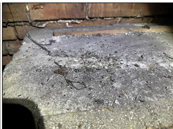
Figure 13: Bat droppings on the tank.
