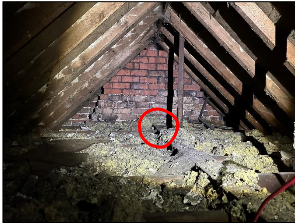
Figure 14: The north of the roof void, droppings circled.
