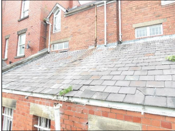
Figure 10: Missing and slipped roof tiles in the extension.
