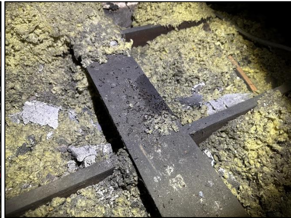
Figure 15: Bat droppings on the loft floor.
