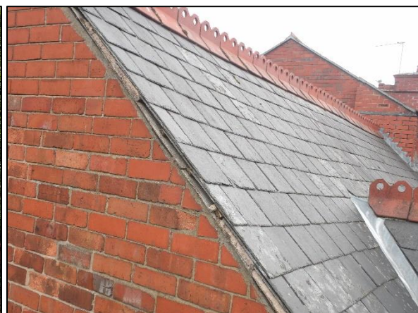
Figure 9: Voids around the verge of the building.
