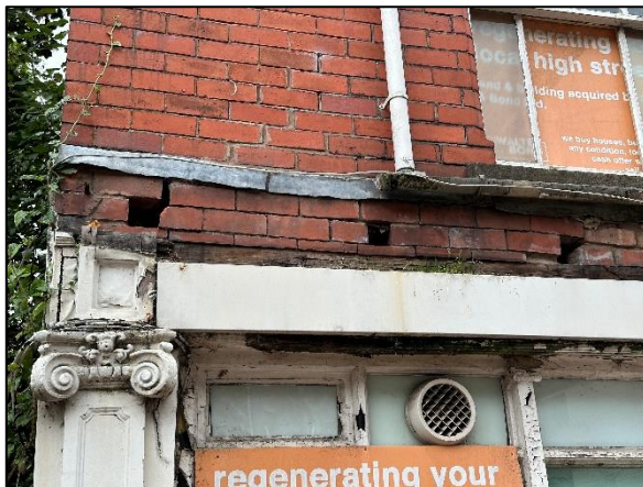
Figure 6: Shallow voids in the western elevation.
