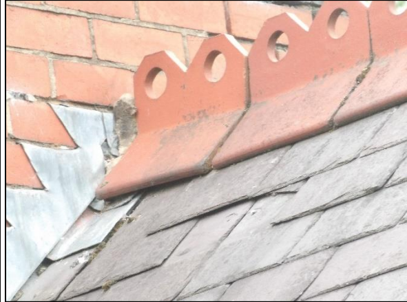
Figure 11: Voids under the ridge tiles of the building.
