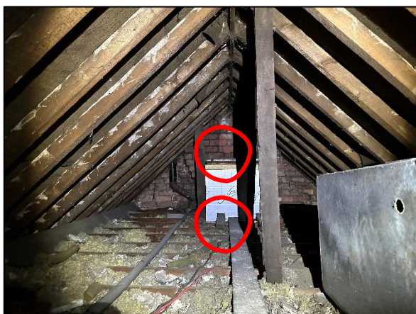
Figure 12: The south of the roof void, droppings circled.
